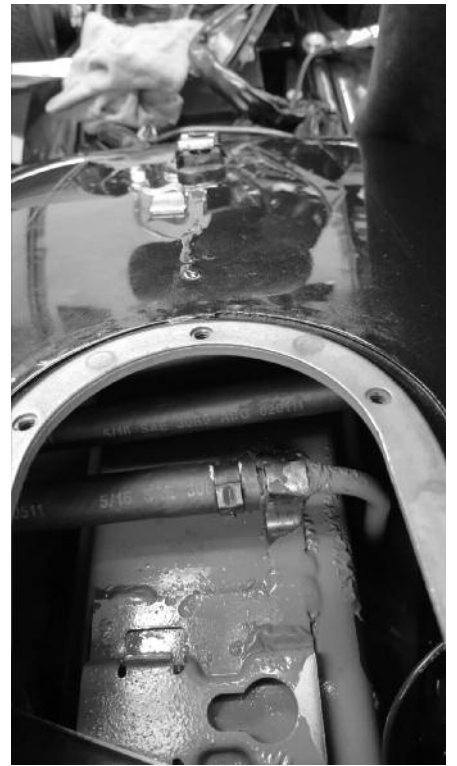
11 After slipping a new clamp onto the last hose to connect, which is the Filter Out hose from the filter, Dan pushes it onto the fitting until it touches the ring on the fitting.
