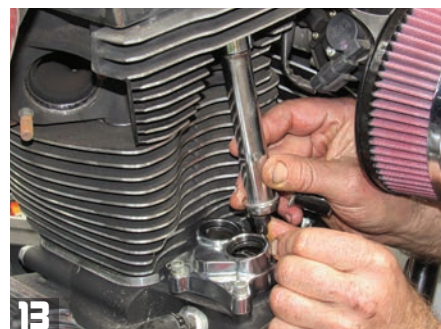
After Dan slips a new Andrews EZ-Install adjustable intake pushrod (there are two intakes and two exhausts) into a stock pushrod tube, he positions the pushrod and tube onto the engine. Next in is the exhaust pushrod and tube.
