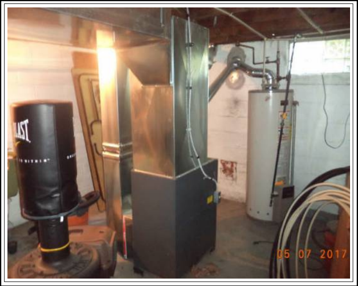
Unfinished basement area mechanicals
