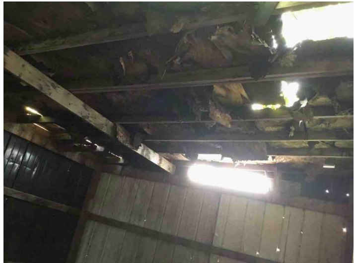
Shed roof requires repair
