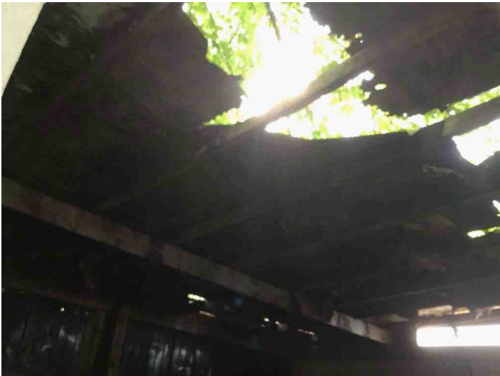
Shed roof requires repair
