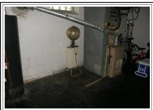
Basement Mechanical Area
