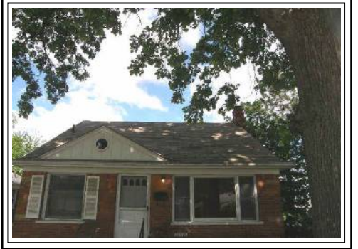
Worn and Weathered Front roof only! The Rear roof in average condition
