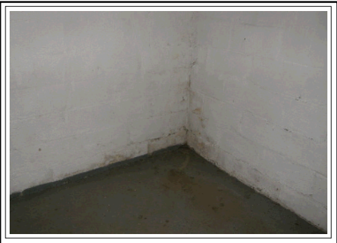
Possible Foundation Issues
