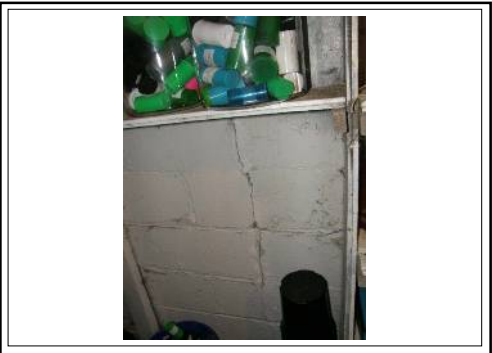
Possible Foundation Issues Foundation Inspection recommended
