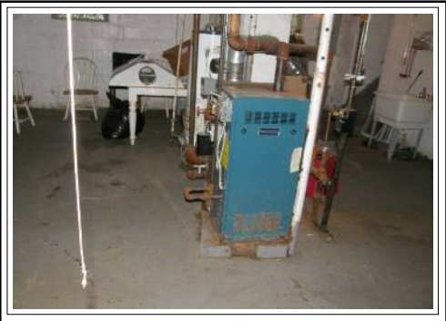
Basement Mechanical Area
