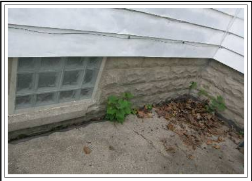
Possible Foundation Issues
