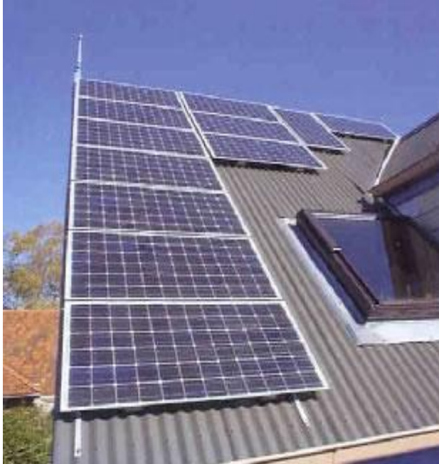
FIGURE 1: ROOF MOUNTED SOLAR INSTALLATION
