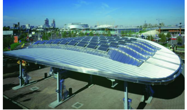
FIGURE 2: LARGE-SCALE PV INSTALLATION (SOURCE – SOLAR CENTURY)
