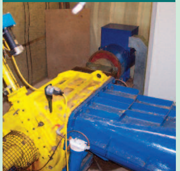
The 90Kw crossflow turbine and generator
