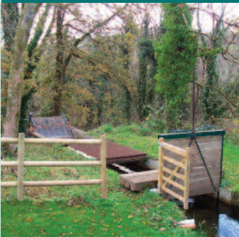
Automatic fish protection and debris screen
