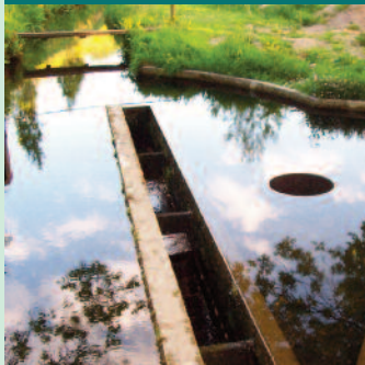
Settlement tank and flood water spillway
